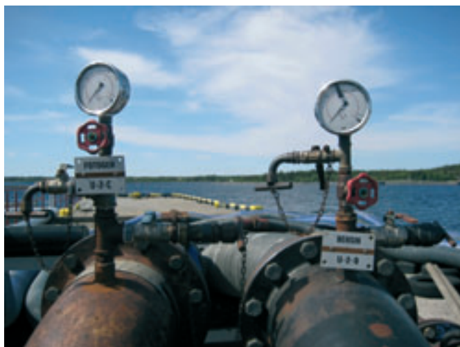
Manometers on the oil dock, with maximum pressure 7 bar marked
