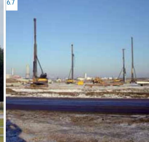
6.6 Third Runway, Arlanda Airport, Stockholm Geotechnical investigations, detailed design of runways, taxiways and drainage systems.
